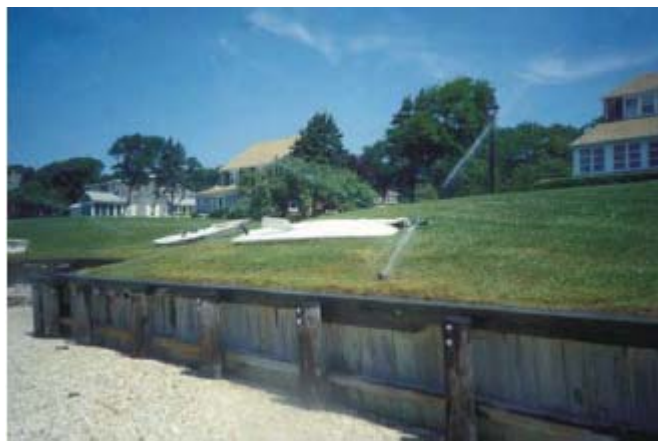
Figure I-8: Wooden Bulkhead as used in NC Sounds
